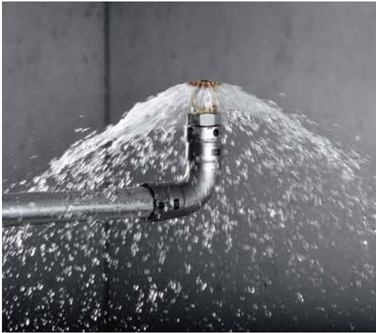
Whether sprinkler unit steel pipes are black, galvanised, painted or powder-coated, Megapress connectors ensure maximum safety.
