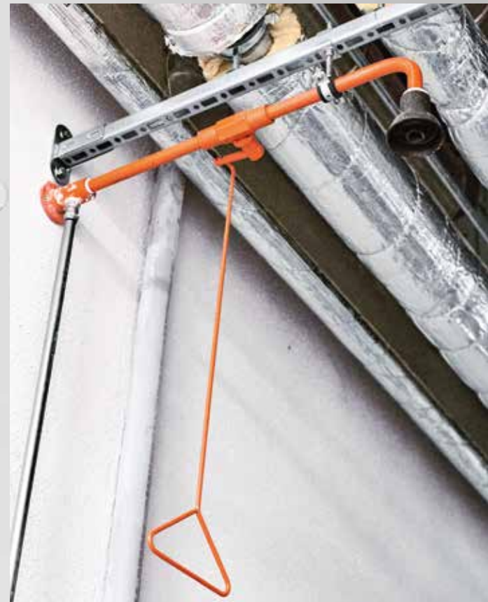
Body shower made with Sanpress Inox in meat product manufacturer Metten's production facilities.
