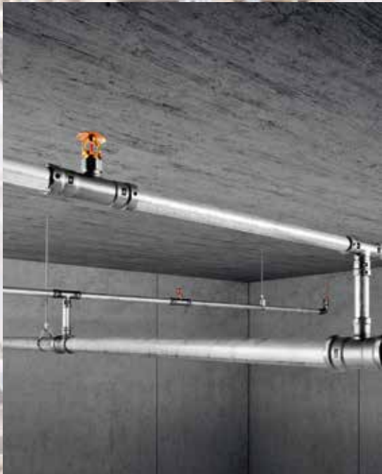
Quick installation of ceiling-mounted extinguishing water pipelines is no problem with Viega piping systems.
