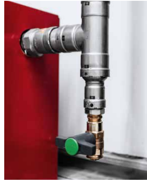
Complying with standards: a fire extinguishing system with Viega press connectors.
