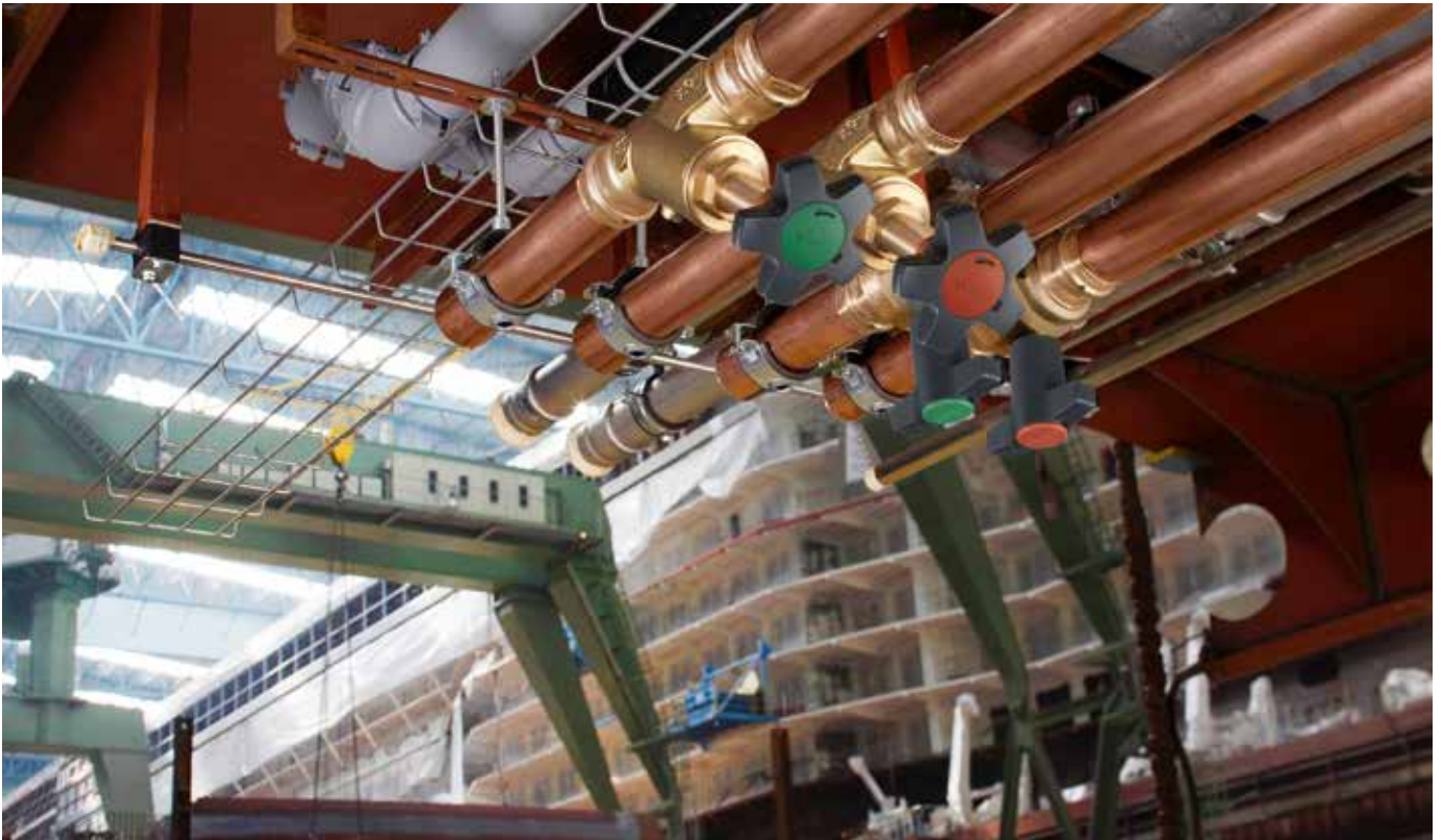
Supporting the construction of ocean-going cruise ships with Viega Profipress and Easytop at the Meyer shipyard, Papenburg.
