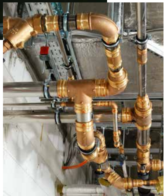
A total of 8 kilometres of Sanpress stainless steel piping was installed for the main drinking water distribution system.
