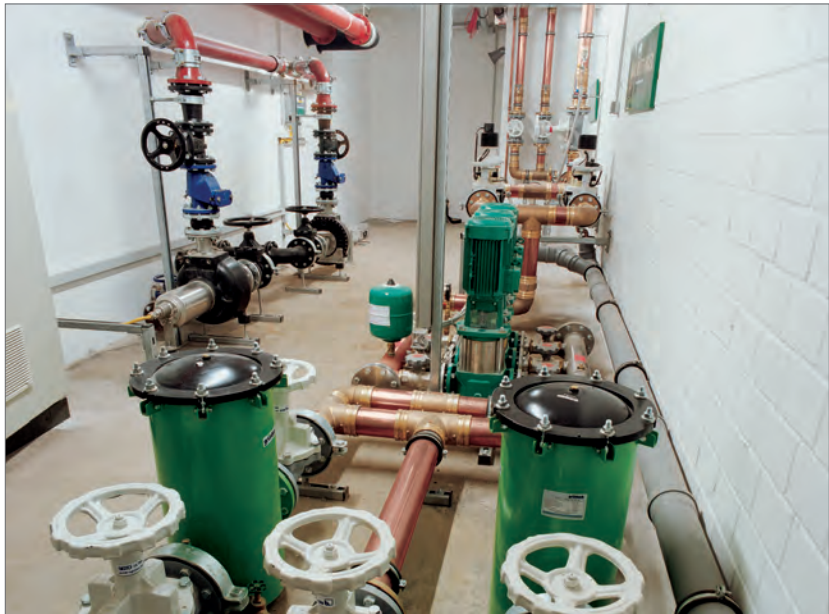
Fig. 173: Treatment system for non-potable water
