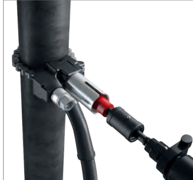
Fig. 37: Next, the hole is drilled by means of a commercially available drilling machine. The steel chips can be extracted by means of the vacuum cleaner nozzle. Afterwards, the holding device is removed again.
