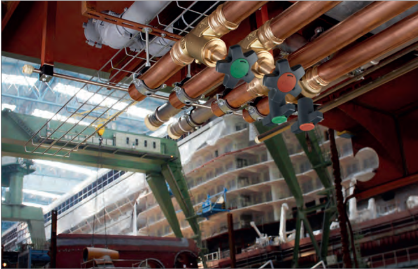
Fig. 178: Copper pipe installations with copper pipes and Easytop fittings
